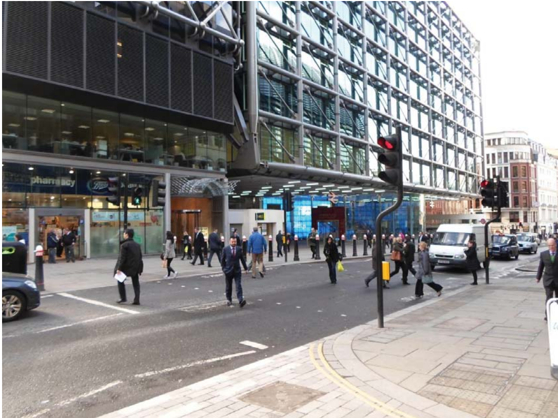
Illustration - Pole installed close to kerb line to avoid utility services. To achieve the necessary 450mm clearance to the signal head a cranked pole was installed.
